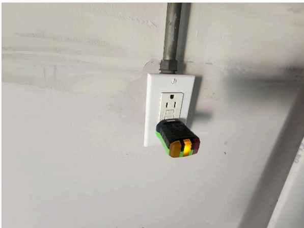
Garage ungrounded outlet
