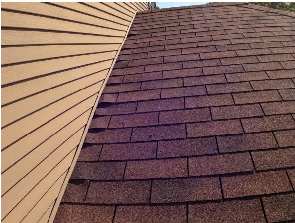
Uplifted asphalt shingles
