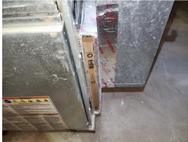
Furnace unsealed filter
