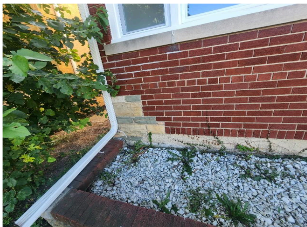
Downspout extension does not extend enough from the foundation
