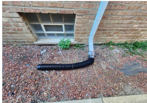
Downspout extension does not extend enough from the foundation
