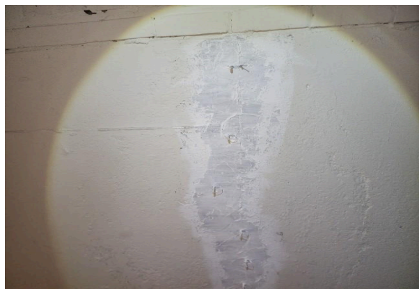
Previous repaired crack in basement wall
