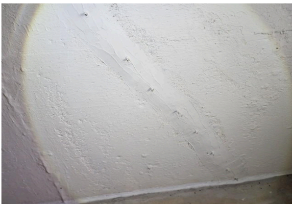
Previous repaired crack in basement wall
